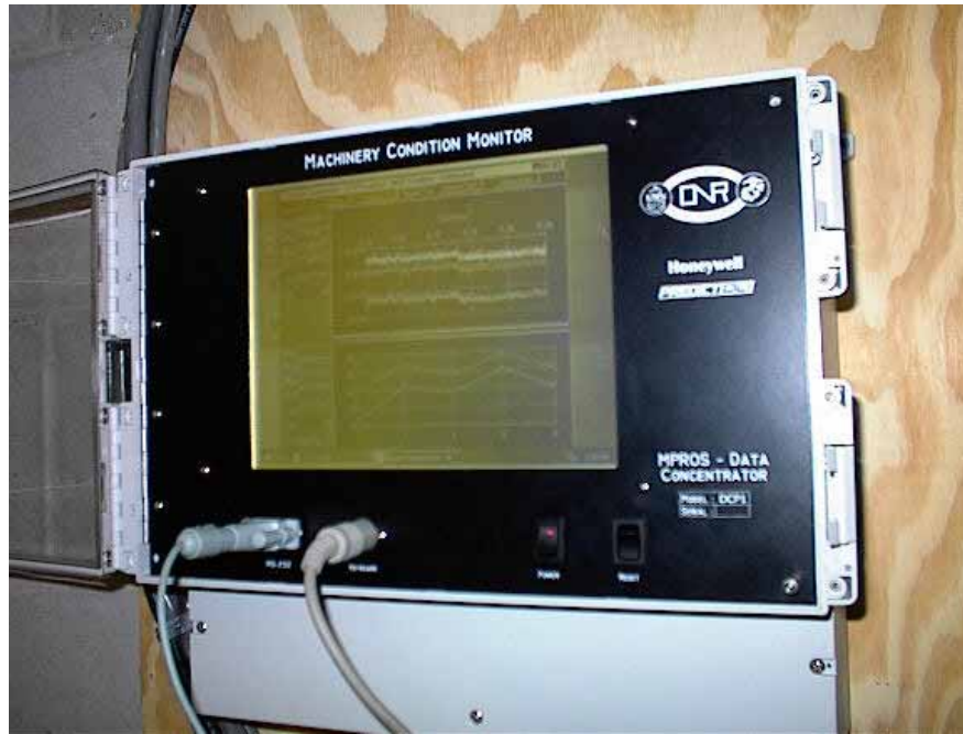
Figure 4. Data Concentrator Installed at HTC
